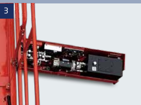
Hydraulic and electric system
